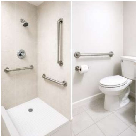
GRAB BARS IN SHOWER & WASHROOM AREAS
